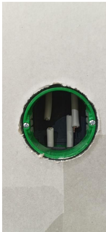
Picture 6. Multifix electrical box installed
